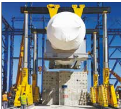
▼ SBL1100 gantry offloading a large generator for installation in a power plant.
