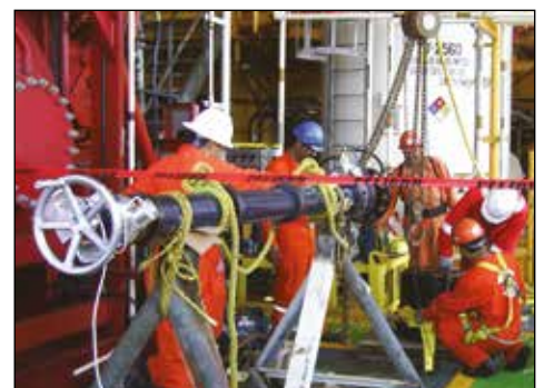
▼ CHT2000 hot tapping offshore application.
